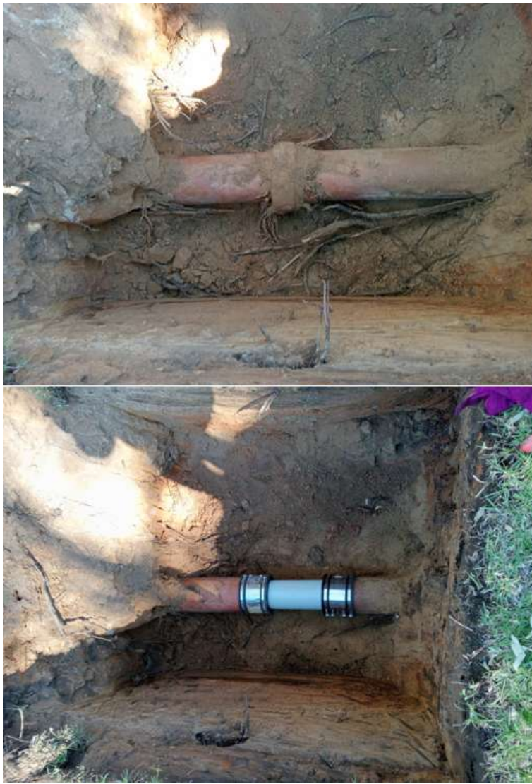
Lone Pine Avenue Corowa sewer service blocked by roots (top) and repaired (bottom)
